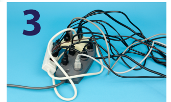
3 Don't use faulty equipment
